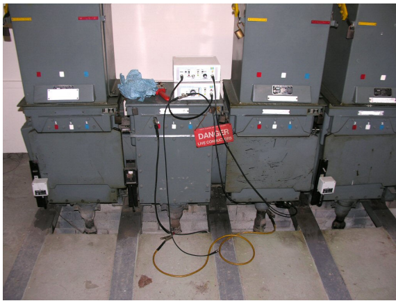
Figure 3 PD location equipment at the far end of the cable
