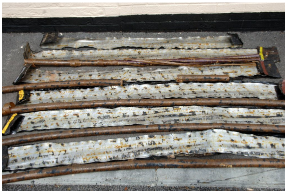
Figure 9 exposed core and lead sheath of around 10m of cable
