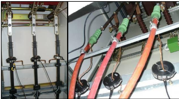
Fig. 3: HFCT sensor attachment inside of switchgear
