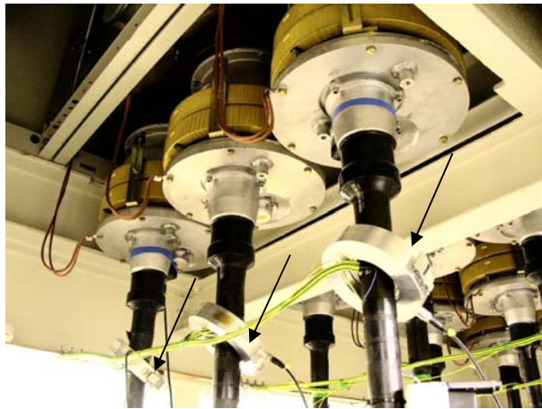
Fig 2 High frequency current transformers (CT's) around cores of 33kV cable for PD measurement (CT's are arrowed)
