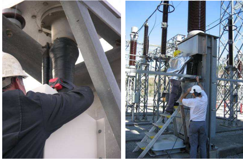
Figure 1 Sensor attachment to 132kV (left) and 220kV (right) cable sealing ends (Note: safety clearances to the exposed high voltage conductors were not breached)
