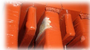
Figure 2. Surface discharge damage on rotating machine end windings
