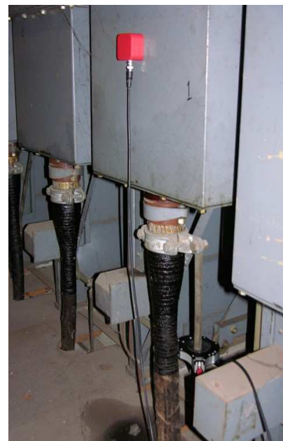
Figure 9: Photo of TEV Sensor Attachment to Cable Box and HFCT connection to Cable Earth Bar
