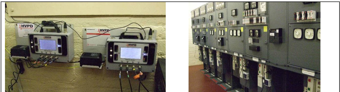
HVPD Mini™ Monitors Installed At Site
