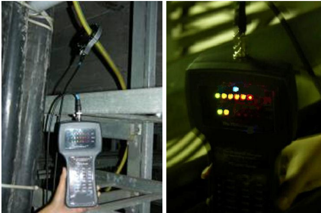
Figure 10: PDSurveyor™ with HFCT on earth strap of N2 Motor Compressor Cable showing 6x LEDs (RED 1 lit) on HFCT (20,000 pC)
