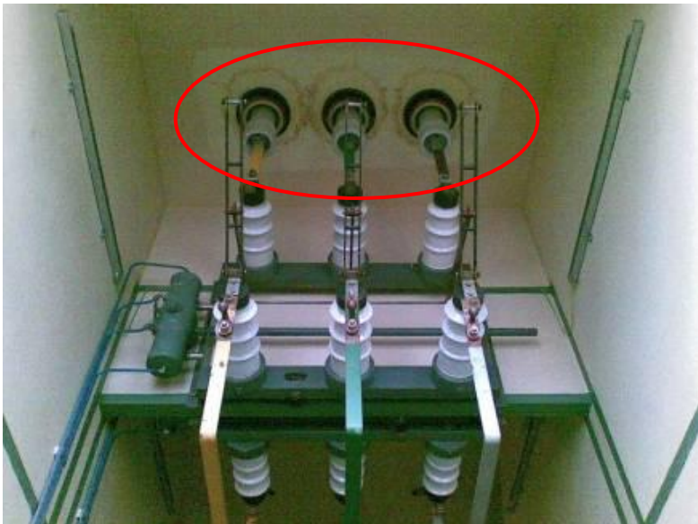
Figure 9: Water Damage on T42 30 kV Bay 2 Bushings
