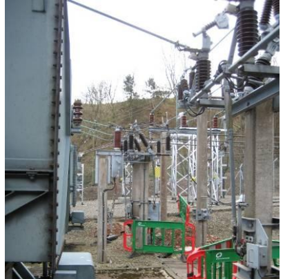
Outside the Substation
