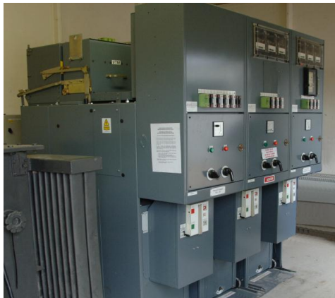
Figure 4: Front View of GEC VMX AIS Panels No.1, No.2 & No.3 (from left to right)
