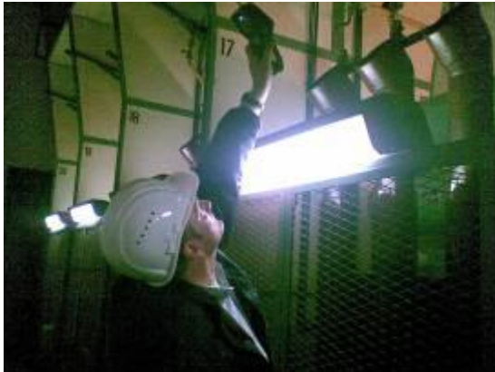
Figure 8: Survey of Air Insulated Switchgear with the PDSurveyor™ Airborne Acoustic Sensor
